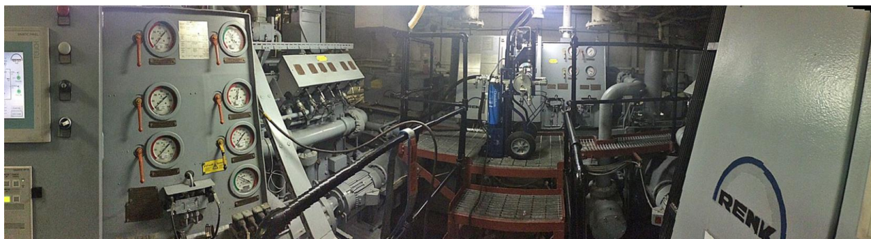
Dehydration system size compared to other hull equipment
