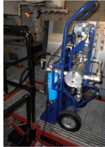
Dehydration system in hull of USGC Waesche
